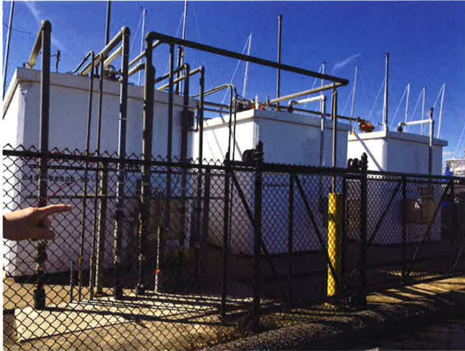
Photo 1: Motor Fuel Aboveground Storage Tanks inside Vault Tanks – inside locked gated
