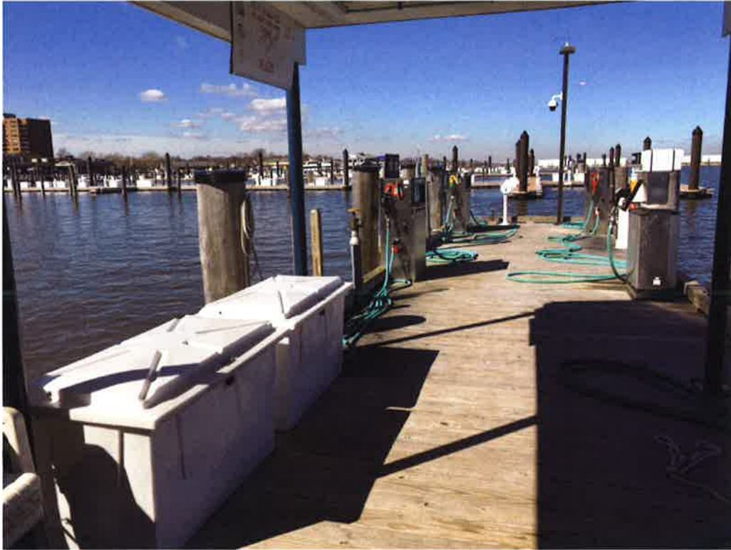
Photo 17: Dock Dispensers and spill kits
