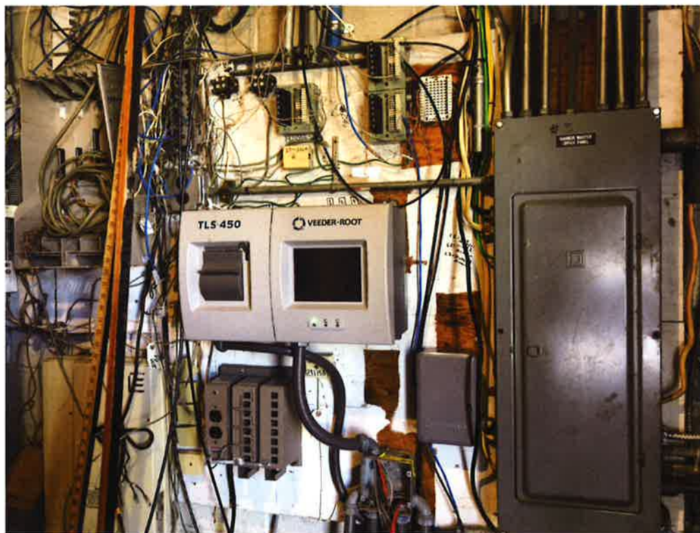
Photo 10: Continuous Monitoring from Veeder Root Systems for Motor Fuel ASTs
