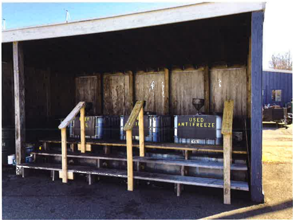
Photo 15: Waste oil tanks in concrete dike
