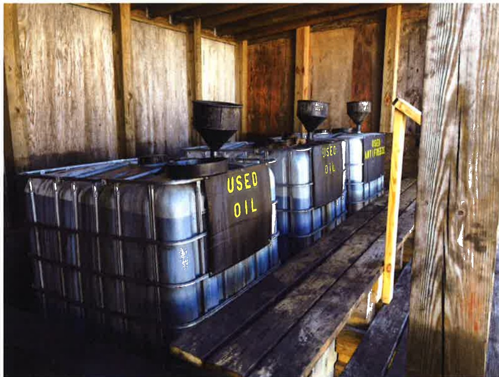
Photo 14: Two (2) 275 Waste Oil Tanks in concrete dike
