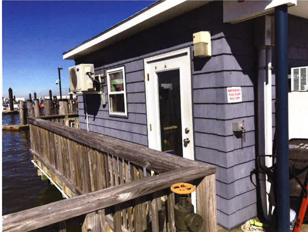
Photo 18: Emergency Shut Off for Dock Dispensers
