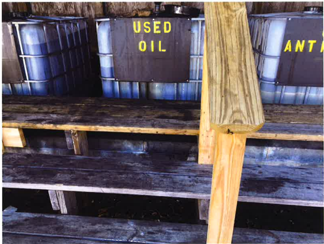
Photo 16: Waste oil tanks in concrete dike
